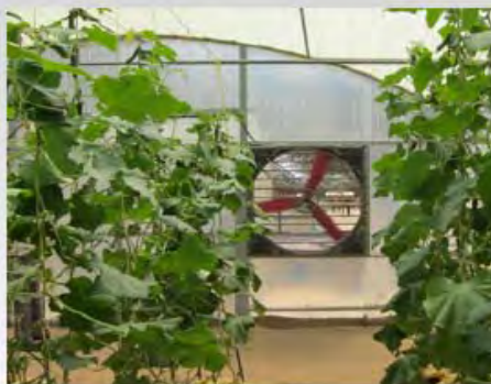
Galvanized Box Fan in Greenhouse
