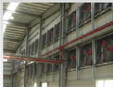
Galvanized Box Fan in Industry
