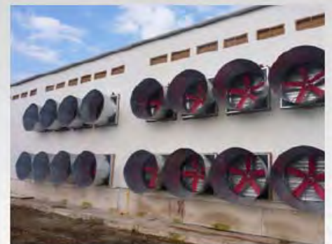
Galvanized Cone Fan in Poultry
